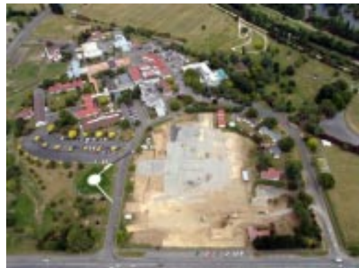
Aerial view showing the footprint of the new hospital taking shape as concrete is poured
