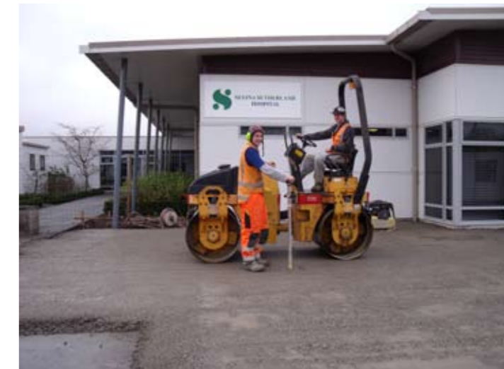
Contactors Marshall Ljestrup and Adam Lister get rolling on the new Selina Sutherland Hospital extension
